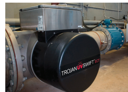
Figure 2. The City of Cornwall, Ontario, Canada currently uses the TrojanUVSwift™ECT to provide year-round primary disinfection and taste and odor removal during intermittent T&O events with a design flowrate of 26.4 MGD (4,164 m 3 /hr).
