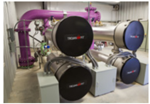
Figure 1. Four TrojanUVFit 32AL50 reactors (2 duty, 2 redundant) installed at Lake Arrowhead's Grass Valley WWTP
